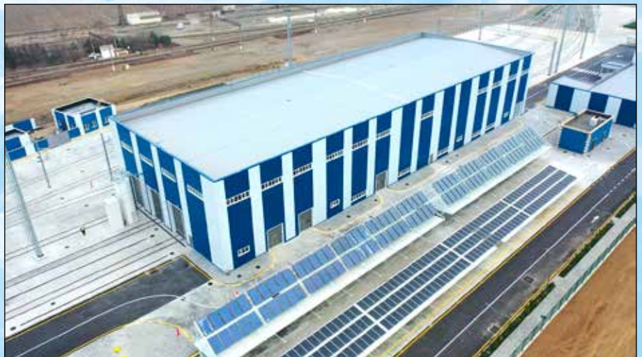
As part of the environmental protection policy, solar panels were installed in locomotive depots in the cities of Bilajari and Ganja
